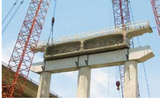
End segments for the main spans were precast on the footing below their final location and lifted into position. Photo: Traylor Bros.
